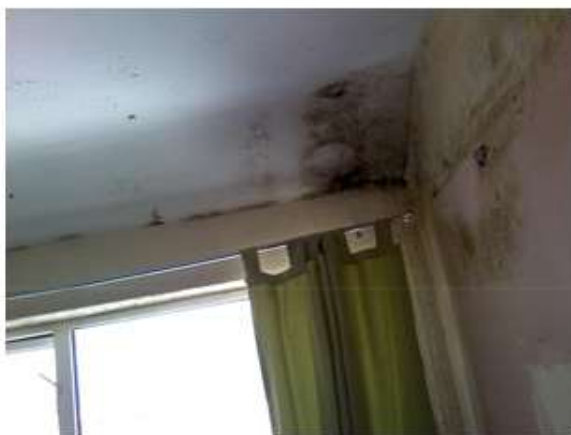
Photo: Wind driven rain penetration damp and black mould
